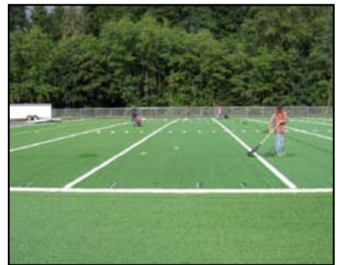
Kellogg, above, and Einstein Middle Schools have beautiful new synthetic turf fields. Work will be completed on all-weather tracks around the fields this month.
